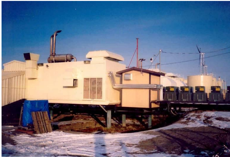
Diesel plant and turbines
